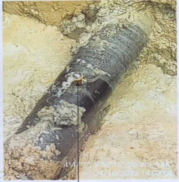
SPILL POINT (INSTALLED 2" VALVE)
